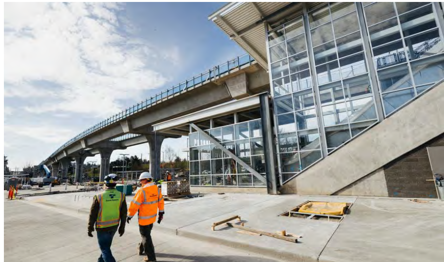
Sound Transit Northgate Link light rail station under construction (Image: Courtesy of Sound Transit)
